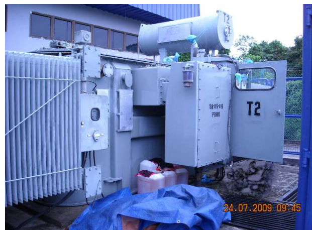
Fig. 1: Transformer under study
