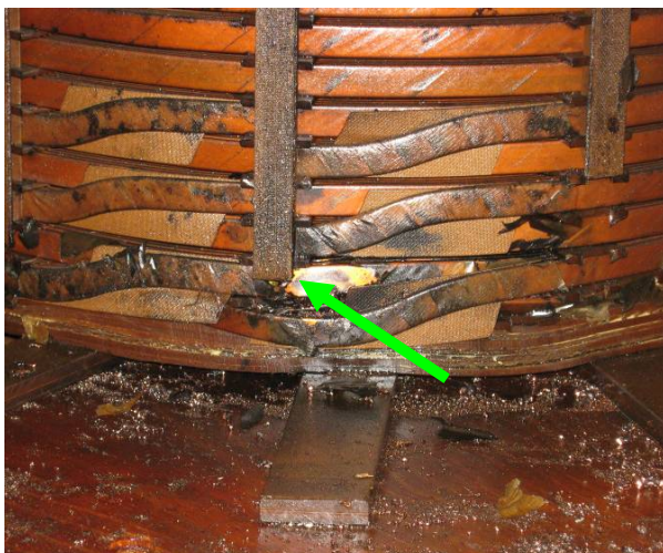
Fig. 12: Arrow shows the arcing spot
