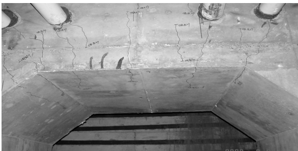
Fig. 3 (a) Actual view of anchor beam cracks
