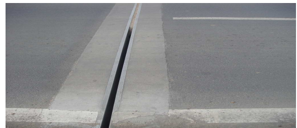
Fig. 4 (b) Losing of joint material
