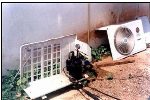
Fig. 3 Photograph of condensing unit of M-AC
