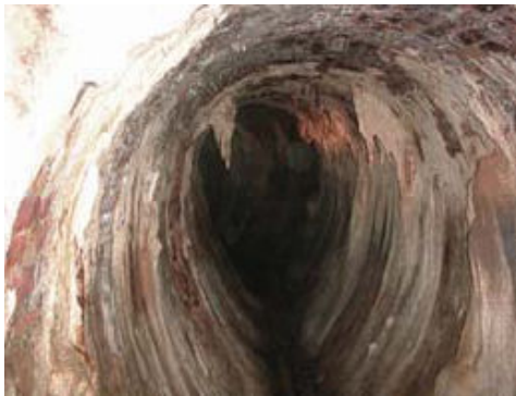
Fig. 9 Obstruction and reduction of the diameter of canalisation of the drainage by sedimentation (weak maintenance)
