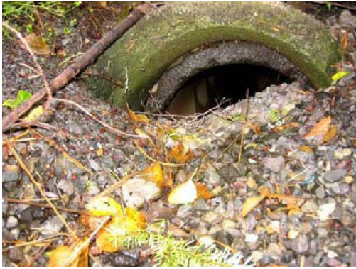
Fig. 8 Obstruction and reduction of the diameter of canalisation. (weak maintenance)
