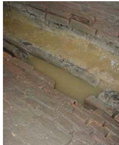
Fig. 7a Deterioration of the bottom of the sewerage canalisation by the velocity of water.
