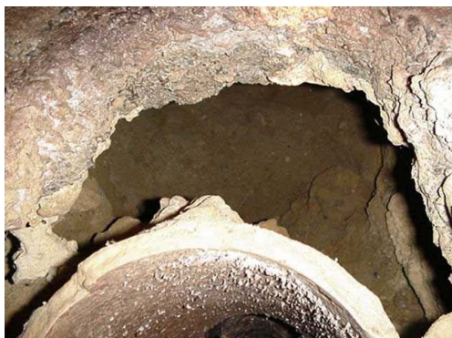
Fig. 10 Delamination of the canalisation by the flood.
